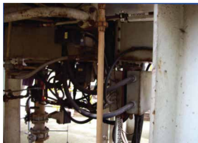
Before: inefficient mechanical system
