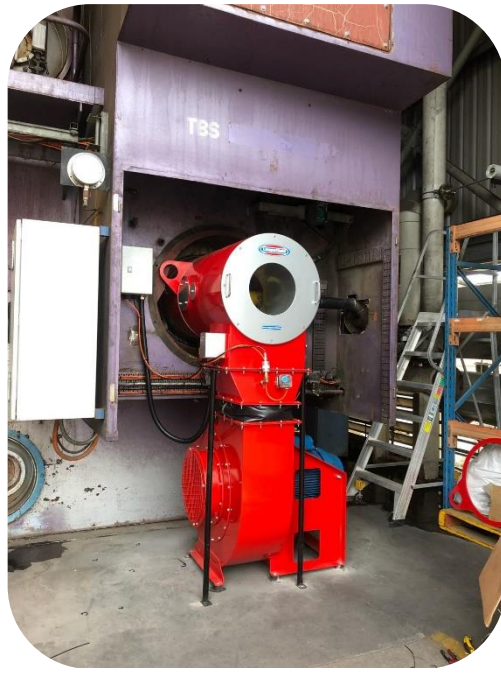
Installed Limpsfield LCN100 Burner at Wetherill Park, Australia, courtesy of CCM Energy Solutions
