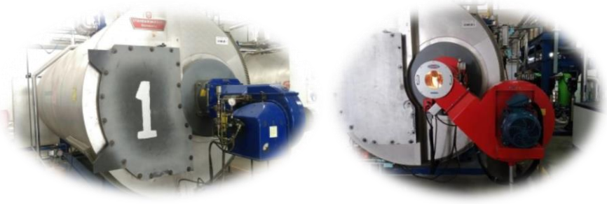
Before (left) and After (right) the installation and commissioning of the Limpsfield LC036 Burner. Photograph courtesy of PASCO.
