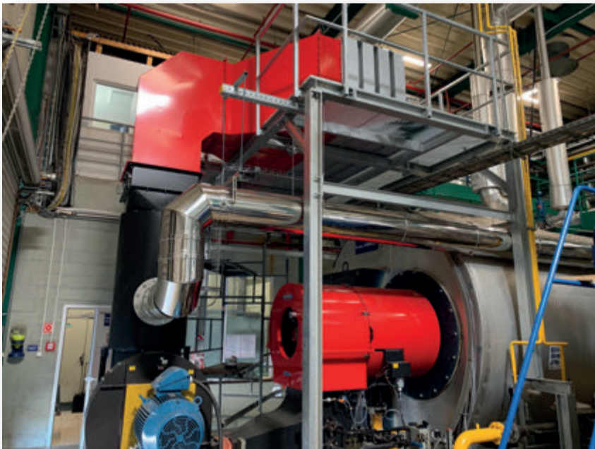
Limpsfield burner designed with FGR + Pre-heated combustion air
