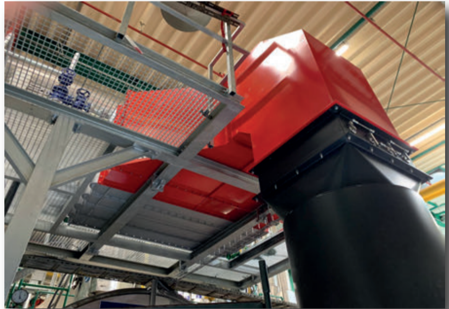
Pre-heated air ductwork connection
