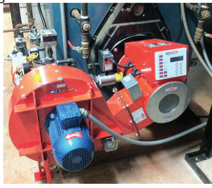
After: Fully modulating Limpsfield burner with precise Autoflame burner controls
