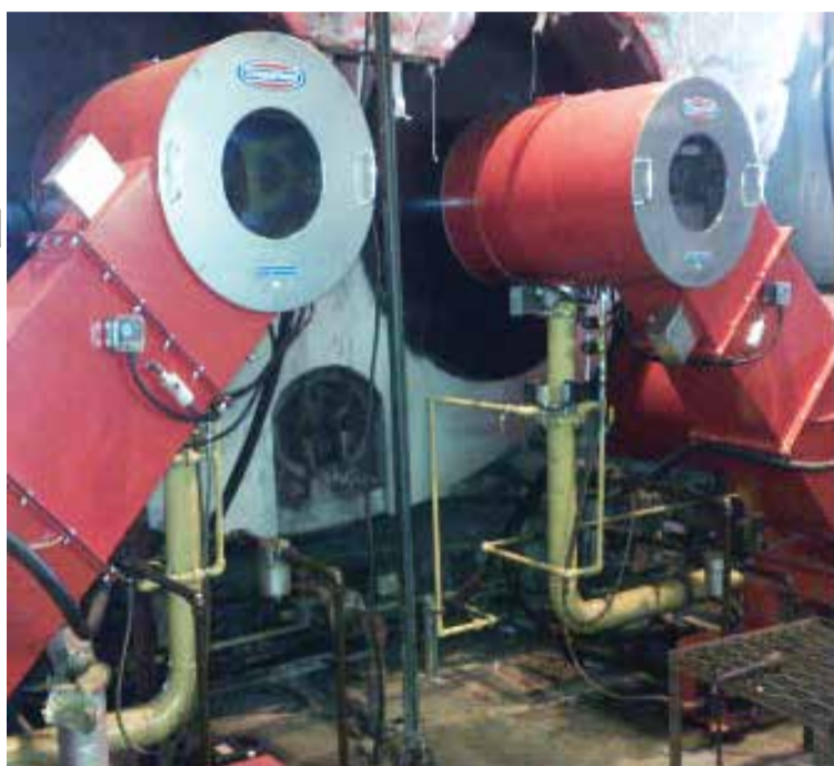
After: Fully modulating Limpsfield burners with Autoflame controls.
