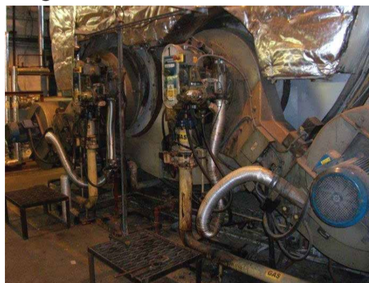
Before: Previous inefficient boiler setup
